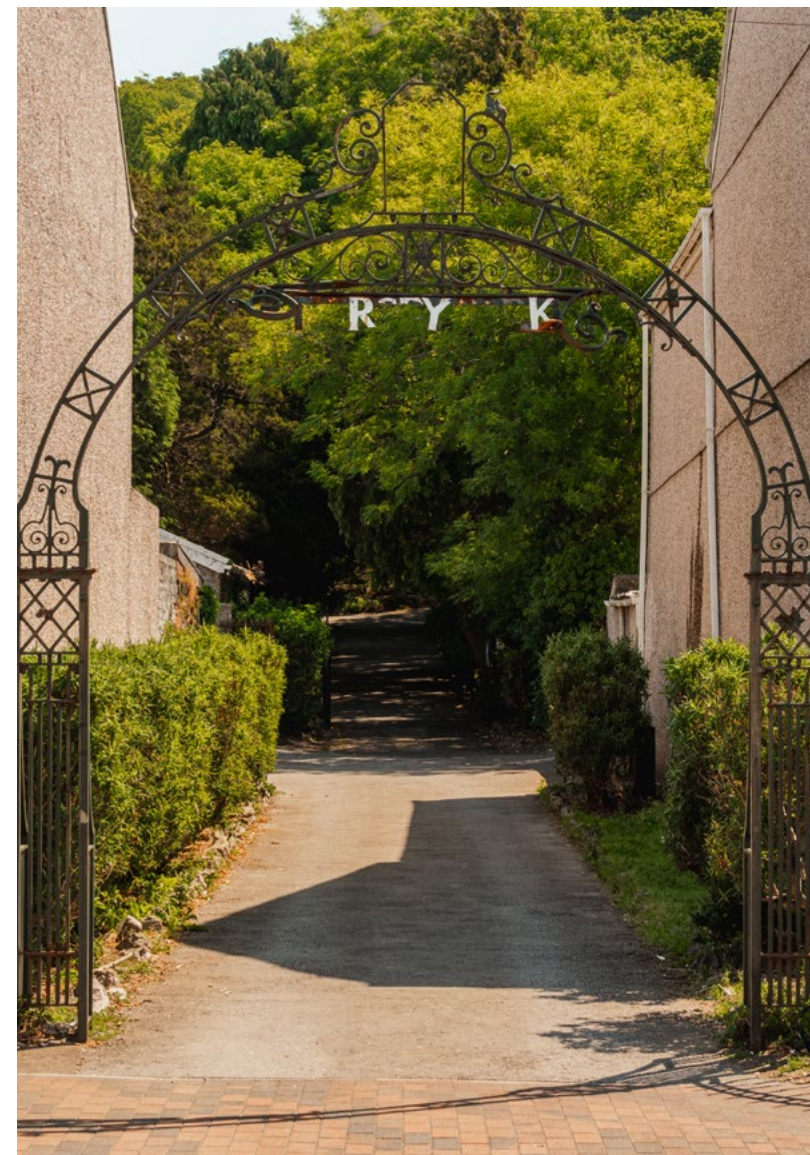
Jersey Park's formal entrance gateway in need of maintenance and repair.
